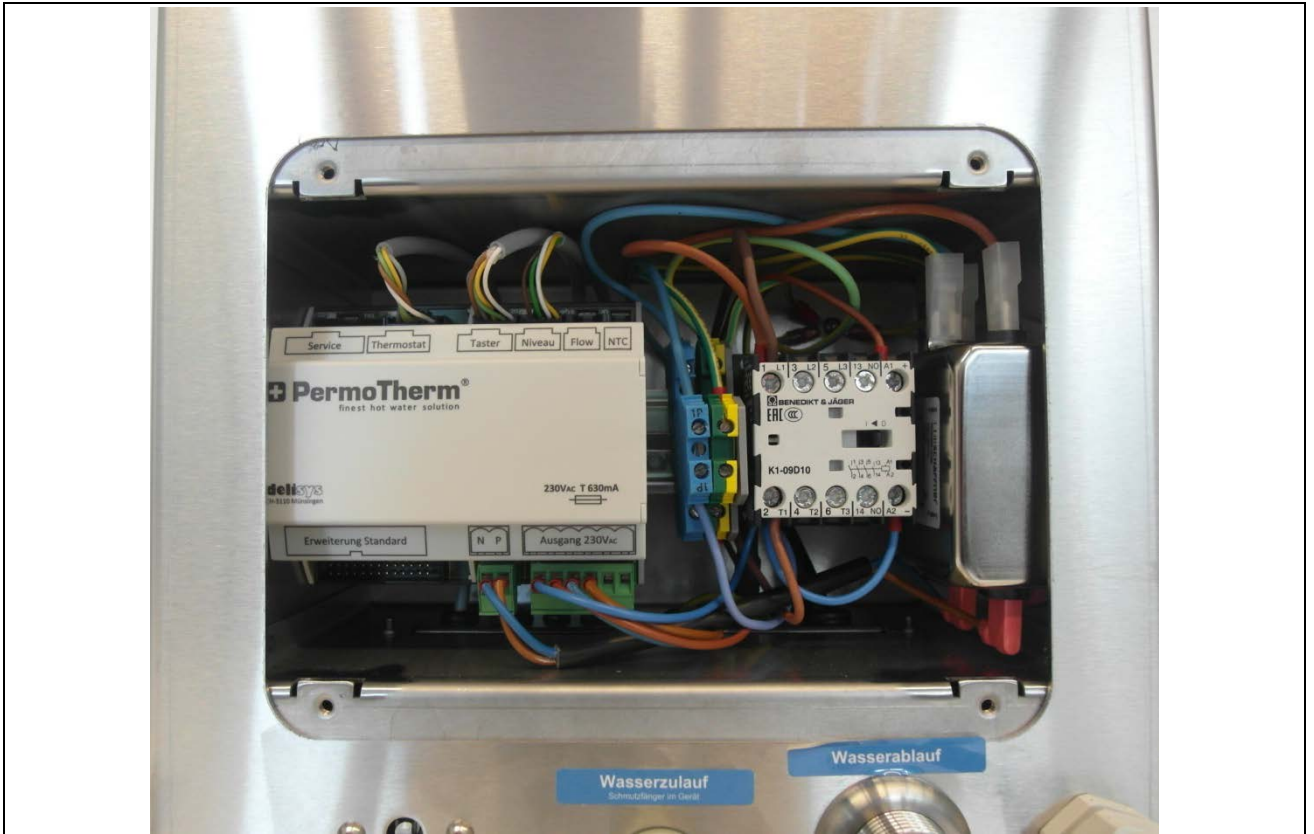
Rear view, cover removed
